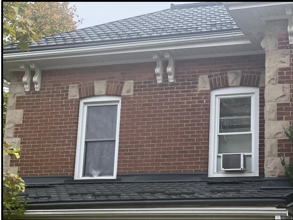
Image 3: Detail of Roofline and Window Openings of 81 Trafalgar Road (Photo taken October 19, 2023; Facing Northeast)
