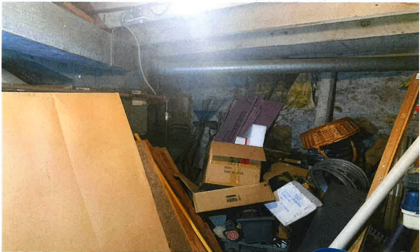
General view of former AST location in the basement of the residential building at 63 Trafalgar Road
