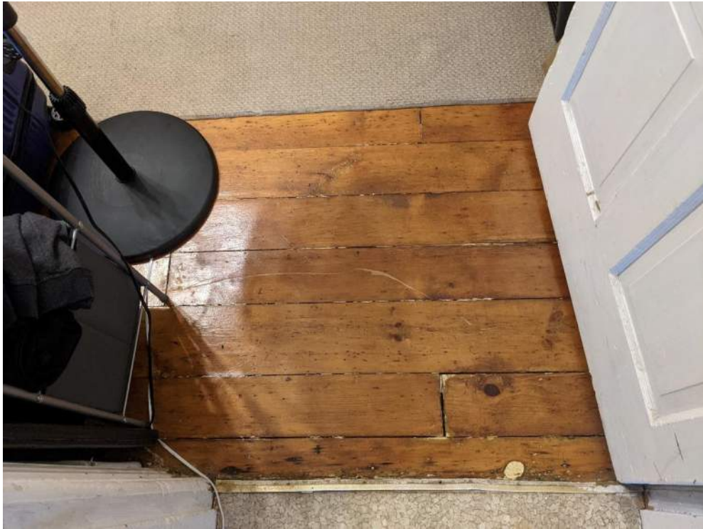
Figure 38: Flooring in rear bedroom/office
