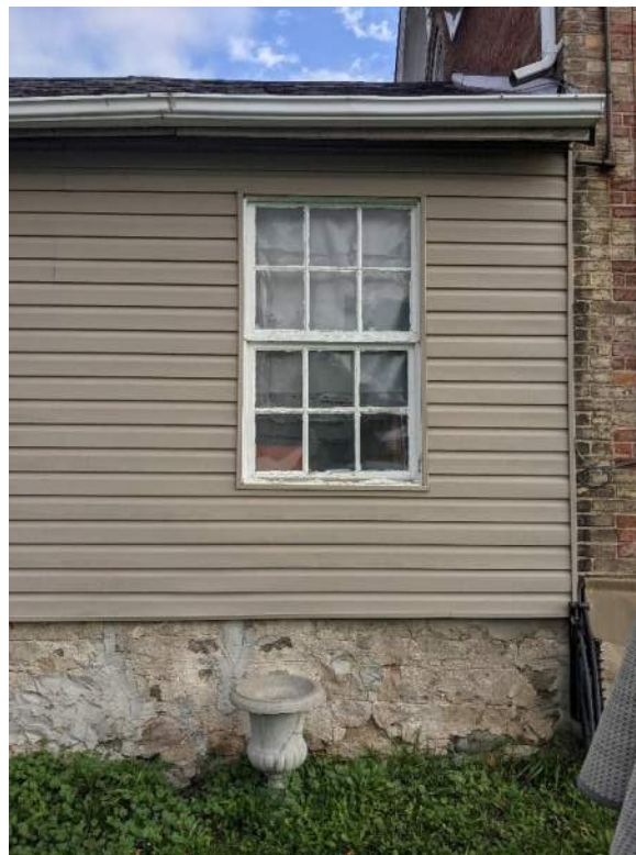
Figure 56: Six over six double hung wood sash window on the west elevation of the north addition
