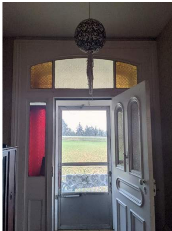
Figure 26: View of the front entrance including wood paneled door and interior transom and sidelights with coloured and patterned glass
