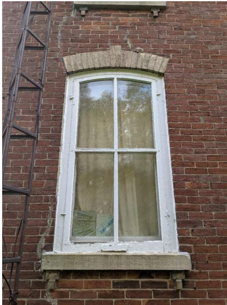
Figure 87: Evidence of cracks radiating around the first and second level windows on the north facade.
