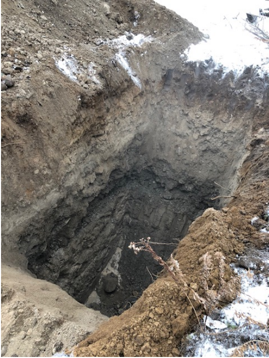
Photograph 15- View of BH 111-water at base was from slow water seepage from sand and gravel seam at 2.4 to 2.8 m below existing grade.
