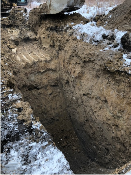
Photograph 3- View of excavation for TP 103. Sides caved in at about 3.8 m below existing grade.
