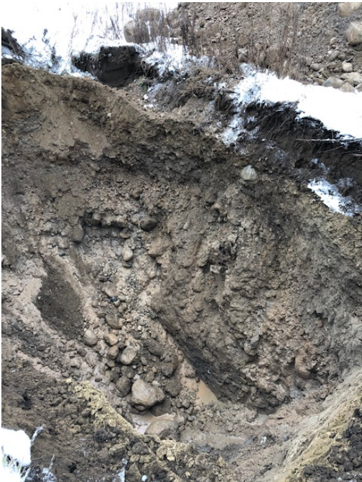
Photograph 6- View of excavation for TP 106. Note fast water seepage from sand and gravel seam at about 2.5 to 3.5 m below the existing grade.
