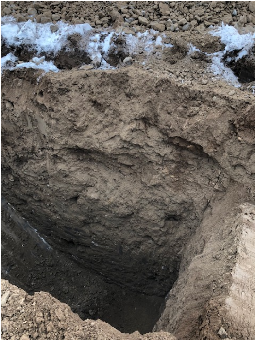
Photograph 4 – View of excavation for TP 104. Test pit was dry upon completion, however after 4.5 hours, slow water seepage was observed at 3.0 m below existing grade.
