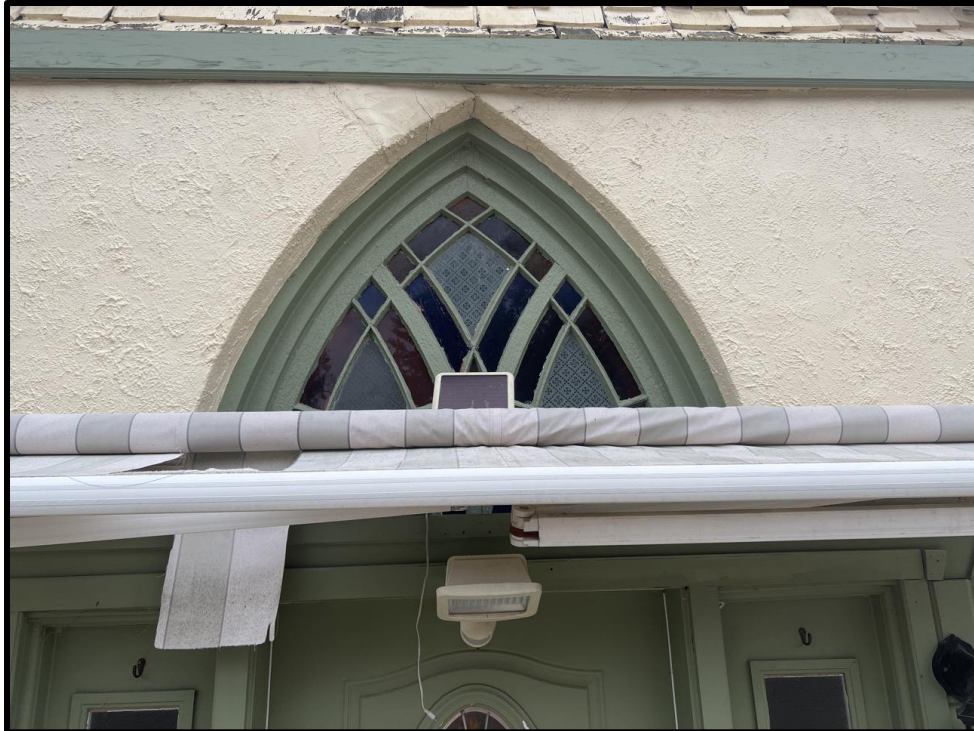
Image 3: Detail of Vestibule Window of 93 Trafalgar Road (Photo taken October 19, 2023; Facing Northeast)
