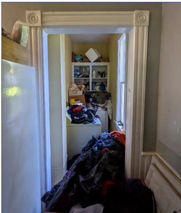
Figure 42: View of the laundry room
