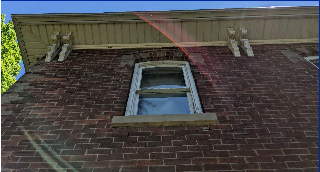
Figure 35: Detailed image of the brackets and a second storey window on the south elevation
