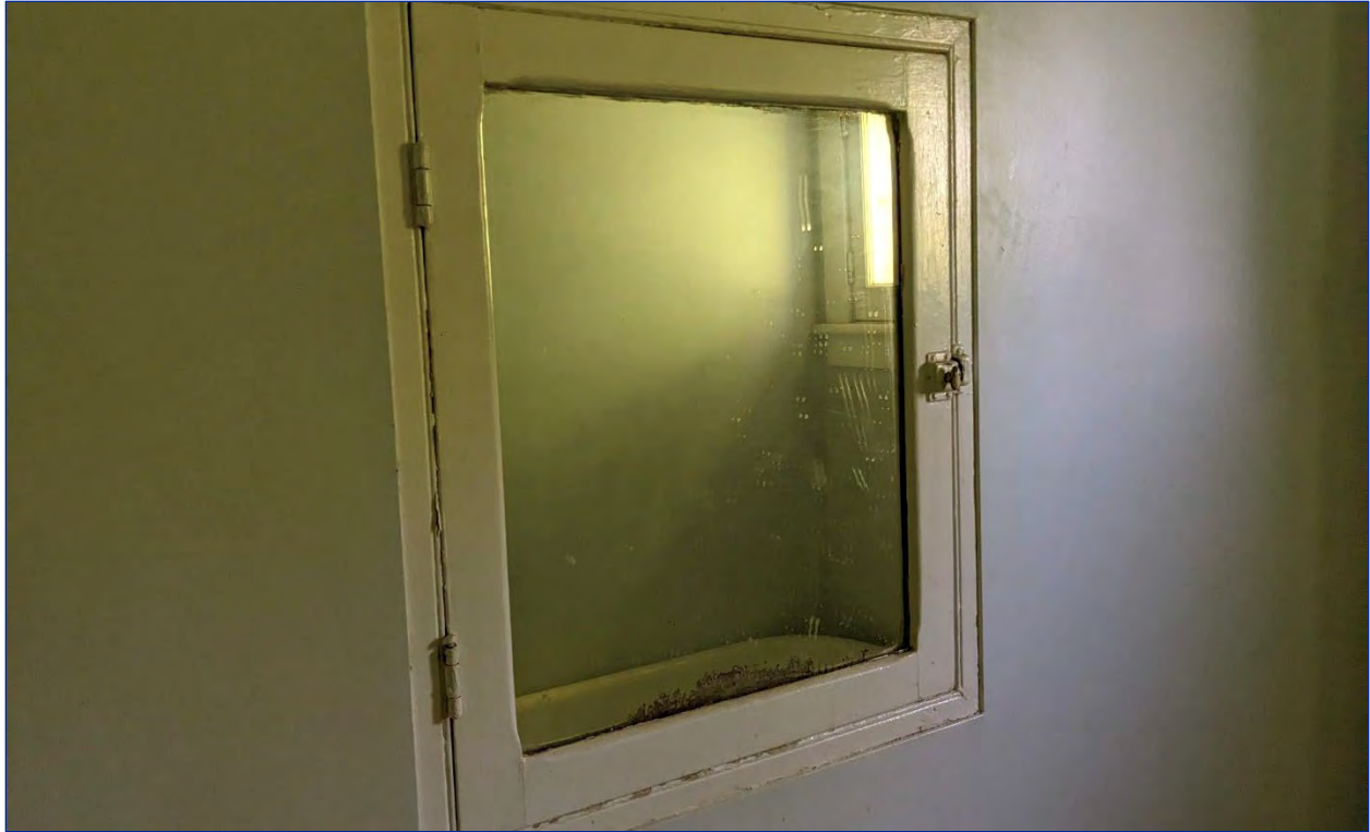
Figure 53: Detailed view of the inset medicine cabinet in the second storey bathroom
