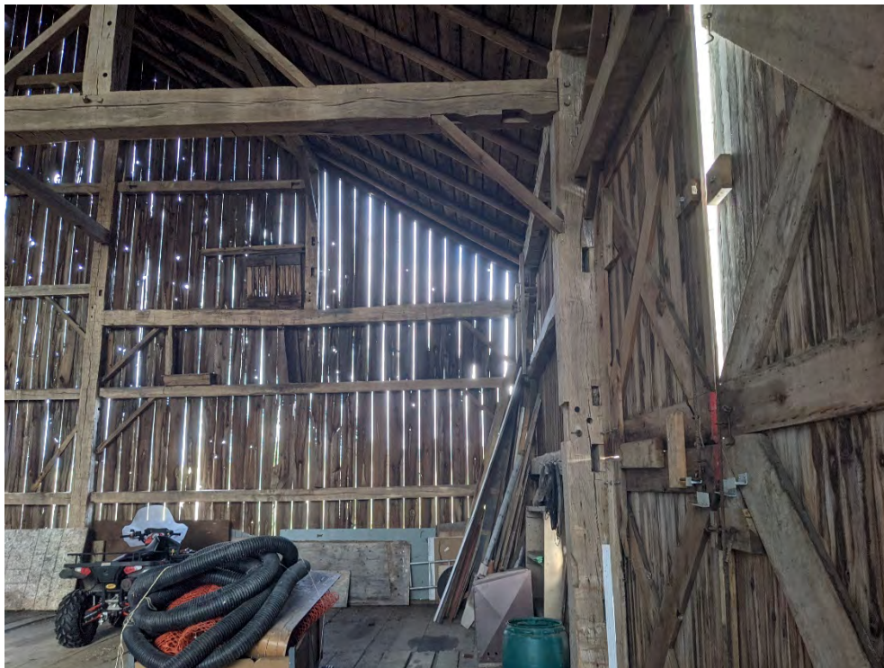
Figure 81: Interior of the large barn, note the extra mortises in the hand-hewn beams
