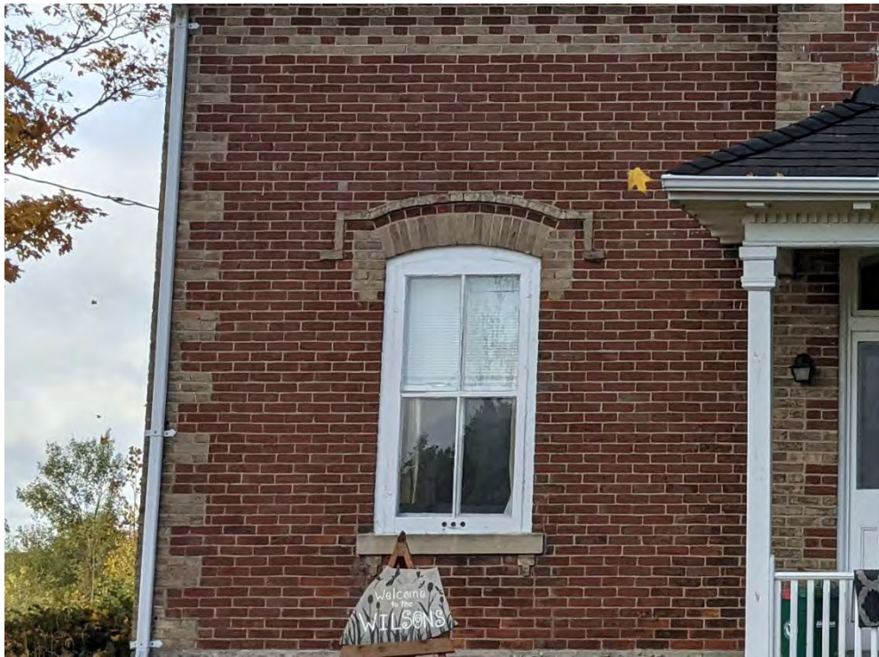
Figure 22: Two-over-two double hung sash window with wood storm door on east façade
