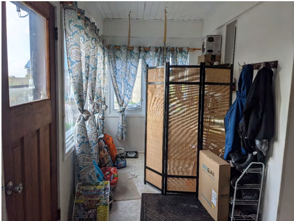
Figure 64: View of the first floor inside the south addition, facing west from the door
