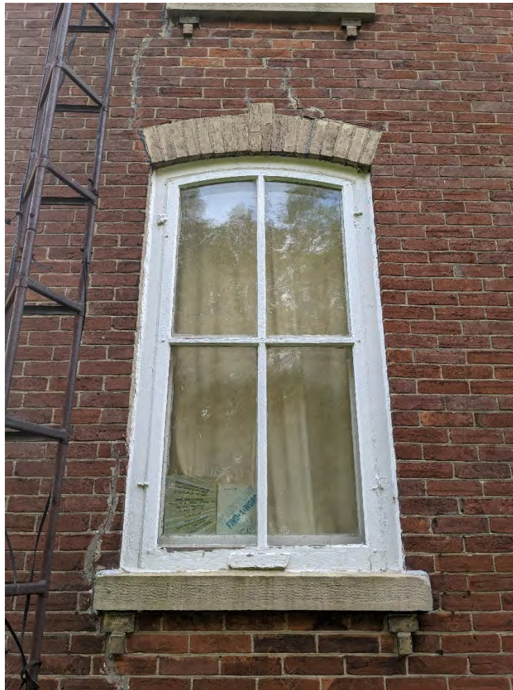
Figure 87: Evidence of cracks radiating around the first and second level windows on the north facade.
