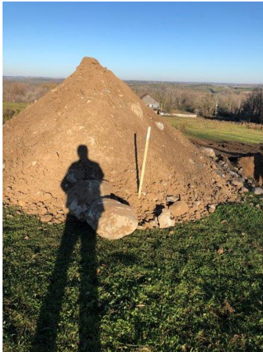
Photograph 12- View of excavated soils from TP11. Note large boulders in soil pile.
