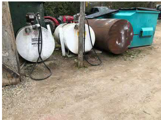
Picture 10: View of the gasoline and diesel ASTs adjacent to the maintenance shop.
