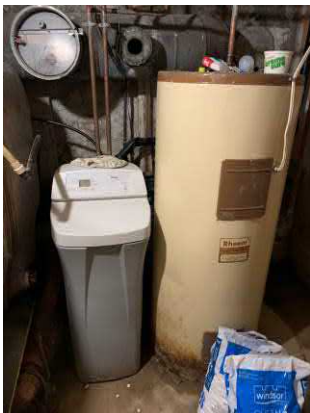
Picture 5: View of electric water heater and water softener in the clubhouse basement.
