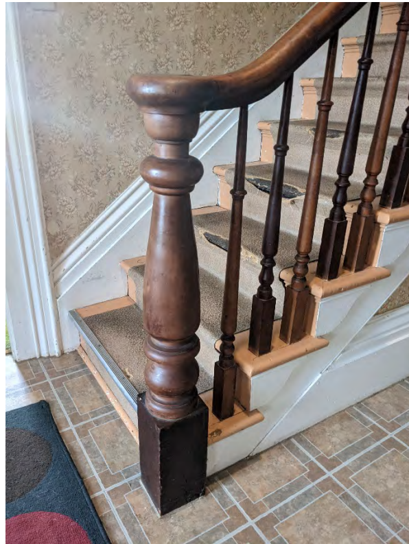
Figure 25: Staircase newel post and spindles
