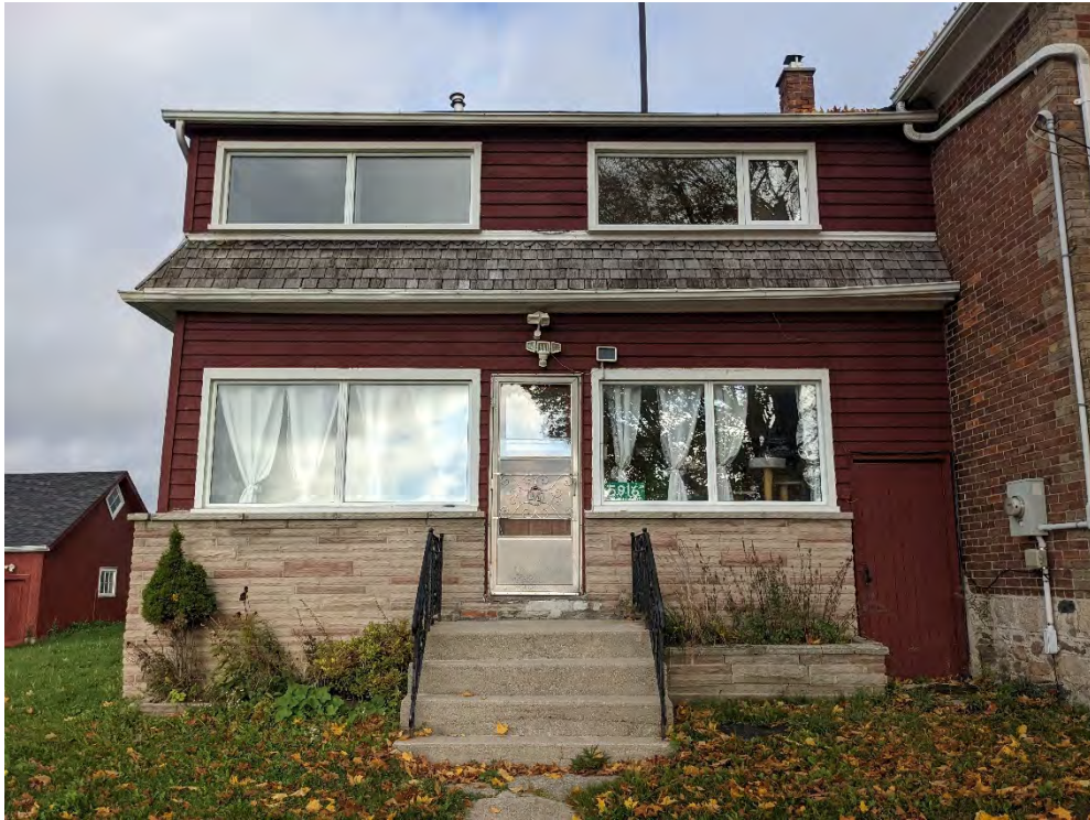
Figure 58: The south elevation of the south addition, note entrance to basement (Right)
