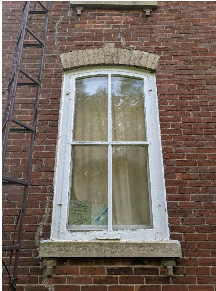
Figure 84: Evidence of cracks radiating around the first and second level windows on the north facade.
