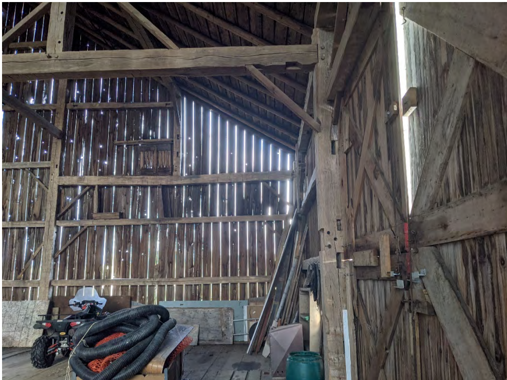
Figure 78: Interior of the large barn, note the extra mortises in the hand-hewn beams
