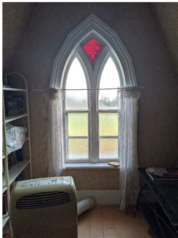
Figure 38: Interior of lancet window on east façade, not coloured and patterned glass in lancet peak
