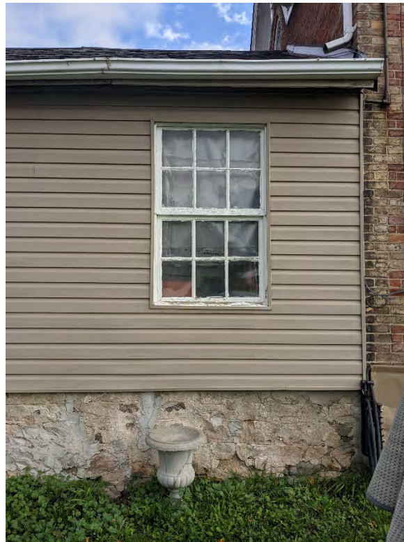
Figure 53: Six over six double hung wood sash window on the west elevation of the north addition
