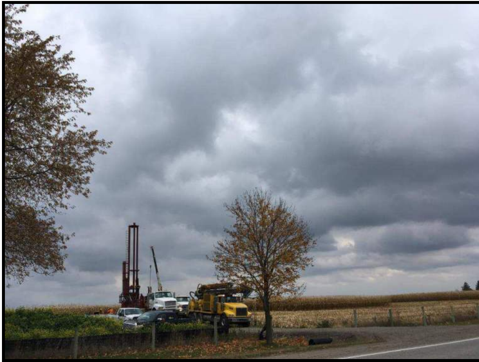
Image 1: View of Erin 3 Well Site, 5657 Wellington Road 23 (October 29, 2019; View Facing East)
