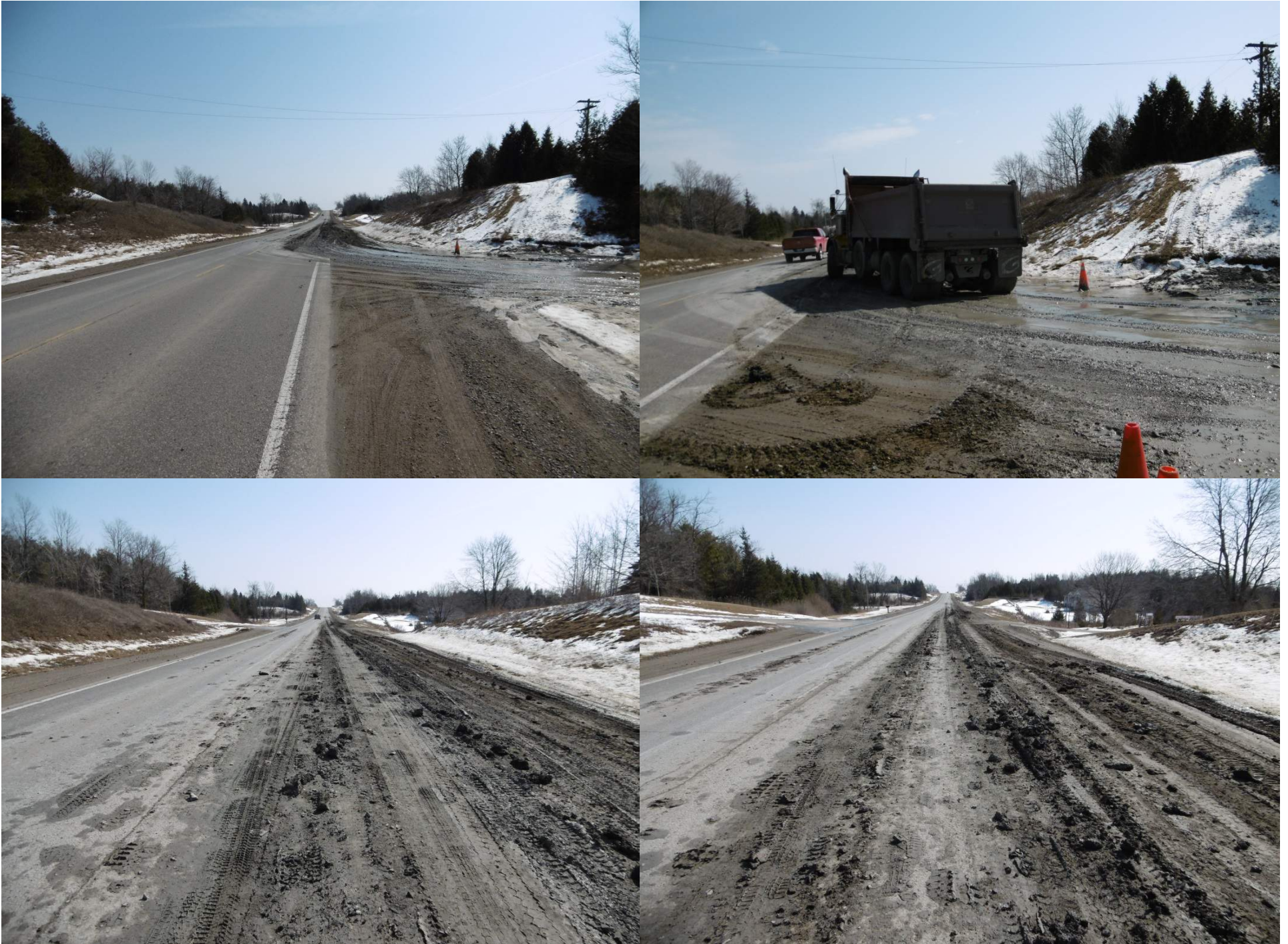
Public Safety Concern: Mud and debris along Wellington Road 125 at entrance to fill operation (Photos taken March 7, 2016)
