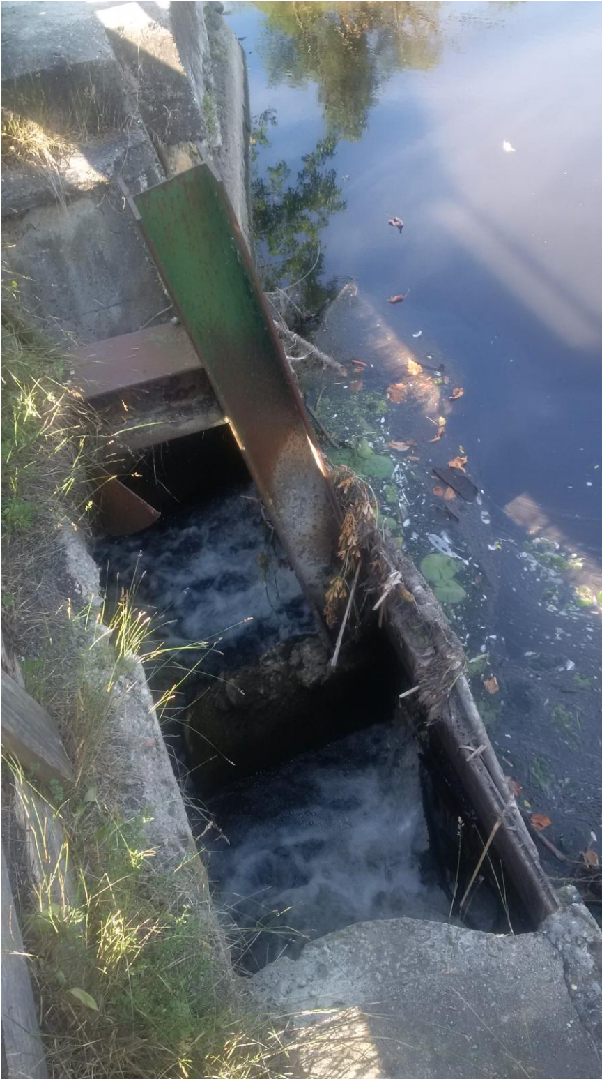
Overhead view of Dam (water passing thru deteriorated boards)
